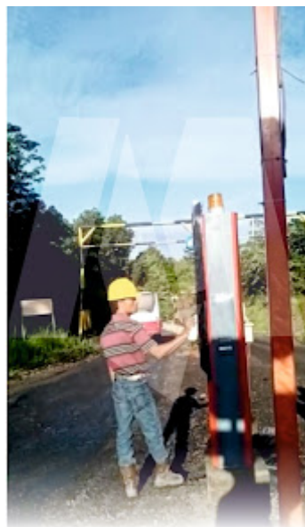
SYSTEM GATE : RFID ONLINE CUSTOM LOKASI PEMASANGAN : PT. MAS LAHAT SUMSEL
